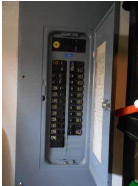
Photo X-6 200 A service panel in garage
