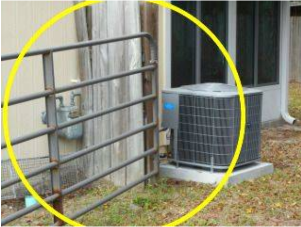
Photo 2-1 proximity of gas meter and AC
