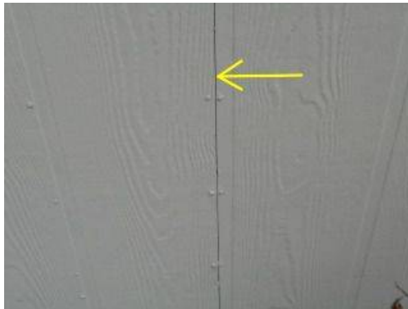
Photo 6-2 Typical shrinkage Hardi panel joints
