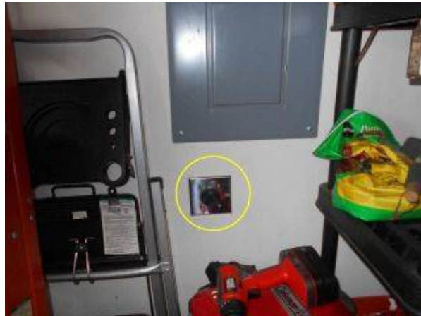
Photo X-2 Aux 240 volt outlet next to main panel in garage
