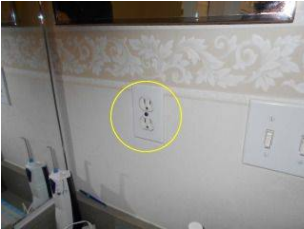
Photo 5-1 M Bath outlet S/B GFCI
