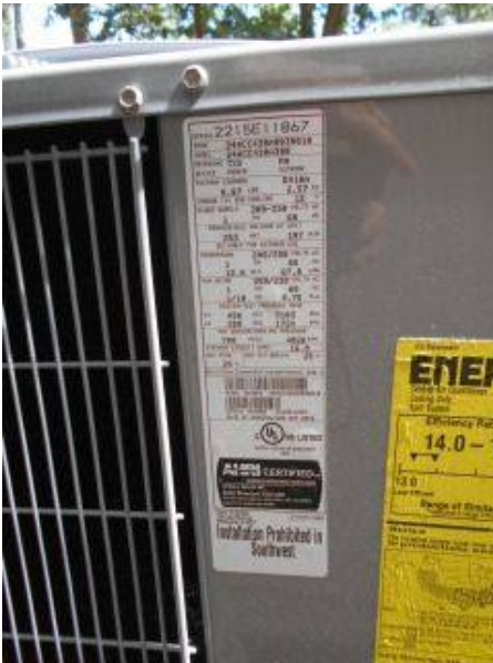
Photo X-1 Carrier 2 yr old compressor unit
