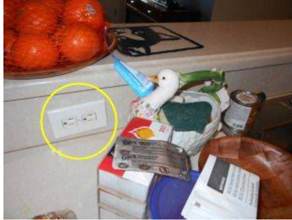
Photo 4-2 kitchen sink outlet S/B GFCI
