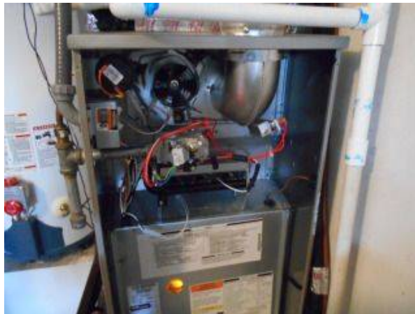
Photo X-8 Natural gas furnace/air handler in garage
