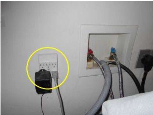
Photo 9-1 Outlet in garage S/B GFCI
