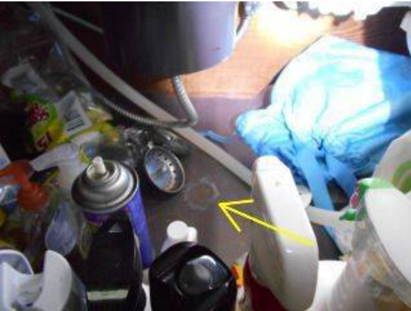
Photo 9-1 kitchen sink cabinet evidence of previous leak now dry
