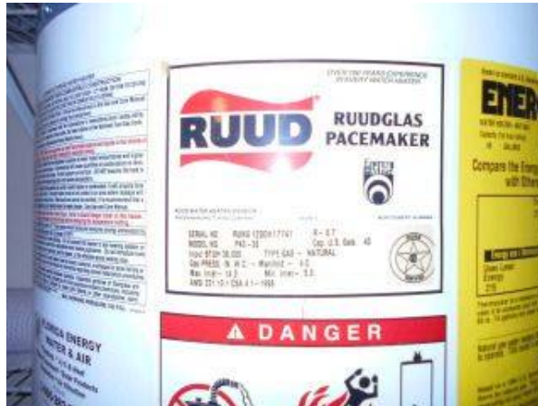
Photo X-12 4 yr old gas water heater working well
