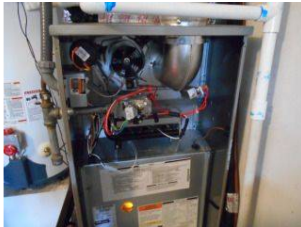
Photo X-8 Natural gas furnace/air handler in garage
