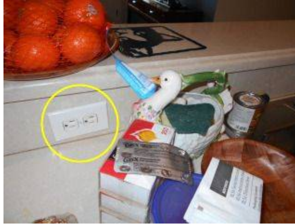
Photo 4-2 kitchen sink outlet S/B GFCI
