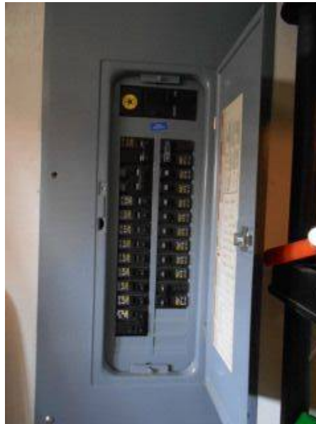
Photo X-6 200 A service panel in garage
