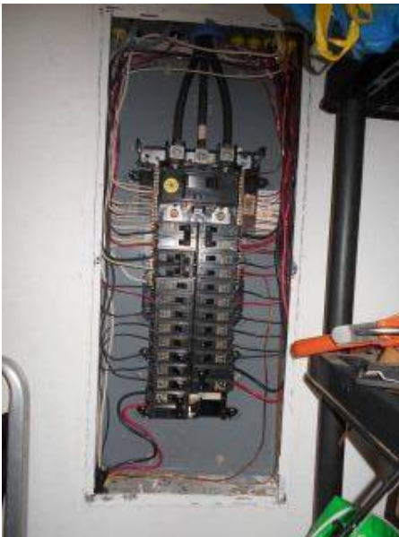
Photo X-7 Main service panel excellent condition
