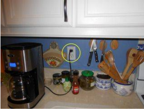
Photo 4-1 kitchen outlet S/B GFCI
