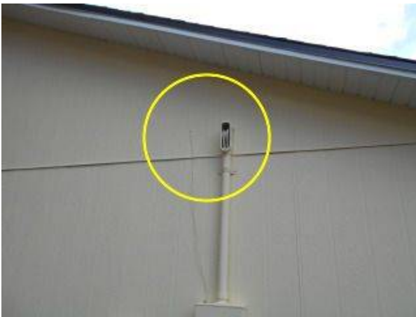
Photo 10-1 missing cover service entrance conduit
