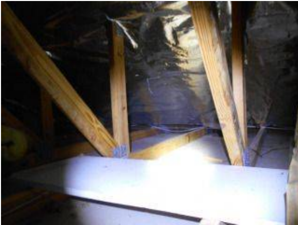
Photo 8-1 insul missing over garage / effective reflective insul on rafters
