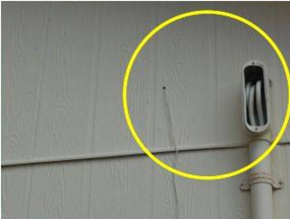
Photo 7-1 missing cover and non caulked telephone wire entry
