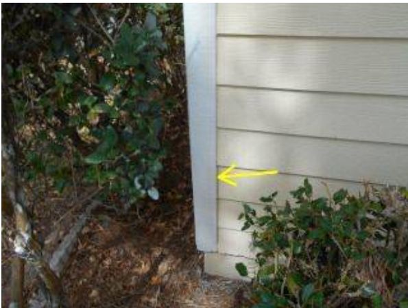
Photo 6-1 shrinkage cracks front siding to trim
